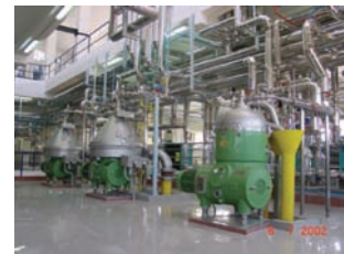
A piping network in an industrial facility
